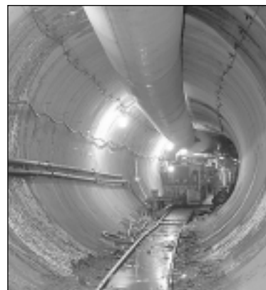
Workers navigate through a section of the newly constructed 17.6-mile MetroWest Tunnel.
