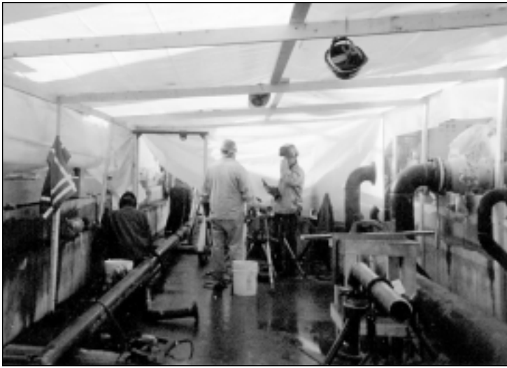
Local 12 members have been piping and welding the MBTA's new liquefied natural gas fueling stations.
