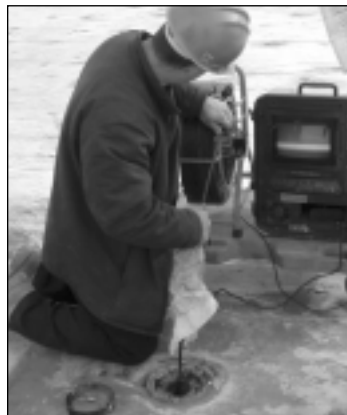
A Local 12 technician from Drain Shooters tests a syphonic drain on the roof of the convention center by inserting a video camera into it. Note the small 2.5-inch pipe size.
